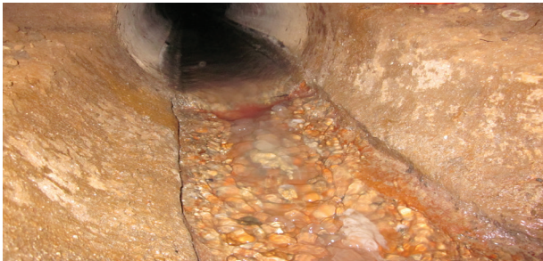
Corroded concrete caused by low pH levels
