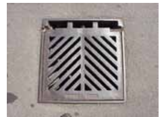
Bicycle-friendly catchbasin cover.
