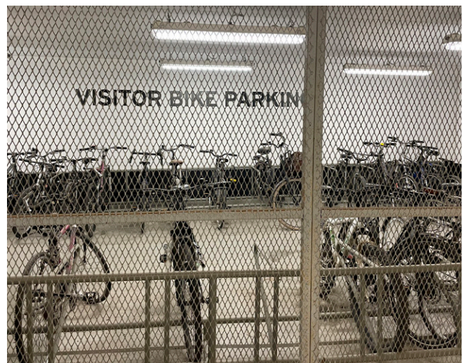
Figure 82. This residential building provides secure storage and parking areas for bikes and mobility scooters.
