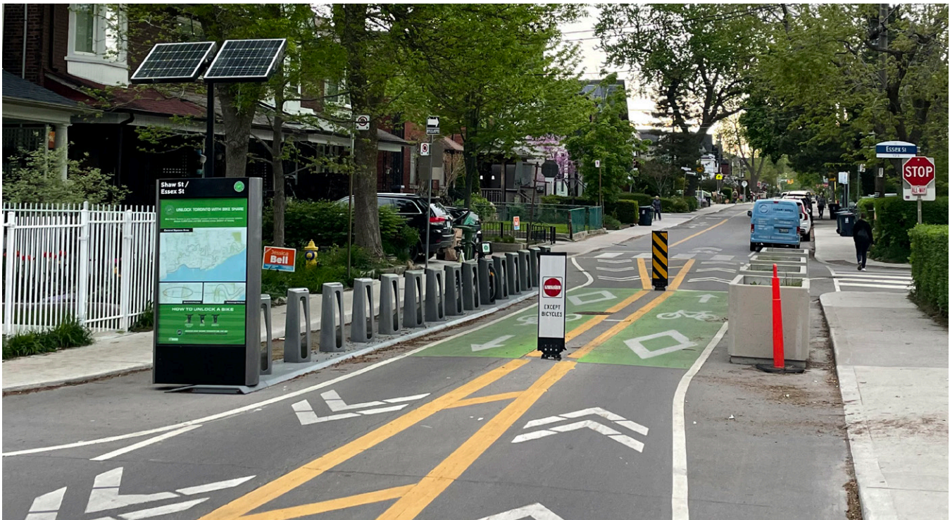
Figure 30. This intervention in the roadway on Shaw Street in Toronto improved safety for cyclists while also calming traffic.
