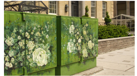
Street art to transform visually disruptive boxes
