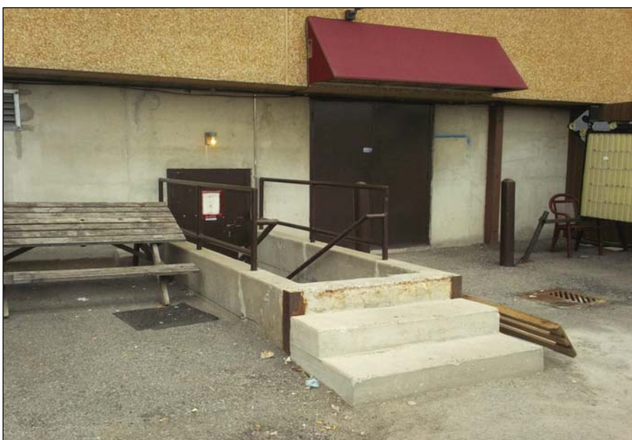
Prevent flood waters from entering low lying building openings
