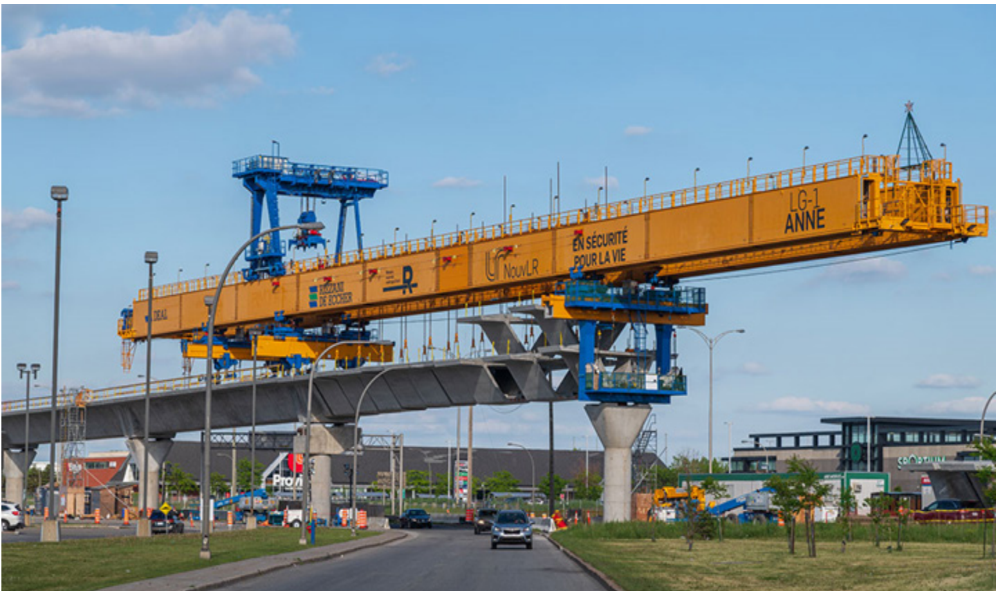
Figure 13. Gantry Crane - Lifts 50 ton of railbed for elevated track on the REM Line in Place
