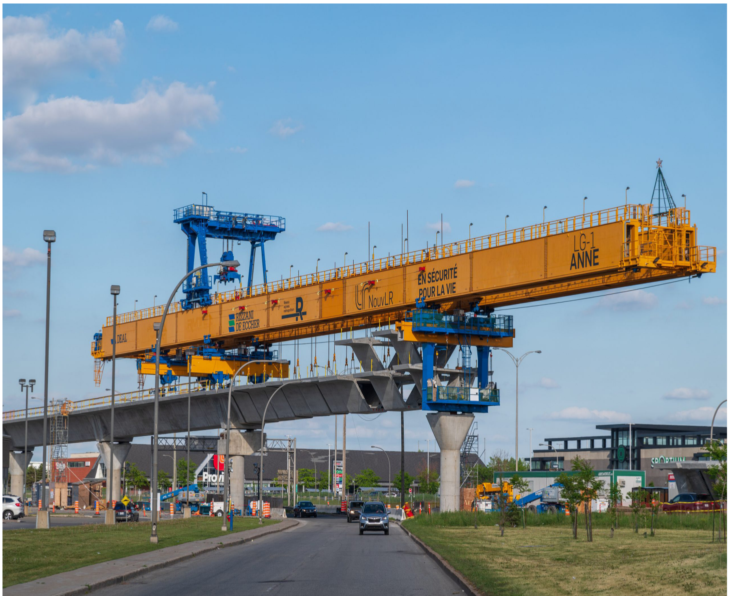
Figure 10. Gantry Crane - Lifts 50 tons of railbed into place for the REM elevated track on the Montreal LRT Line at a time.
